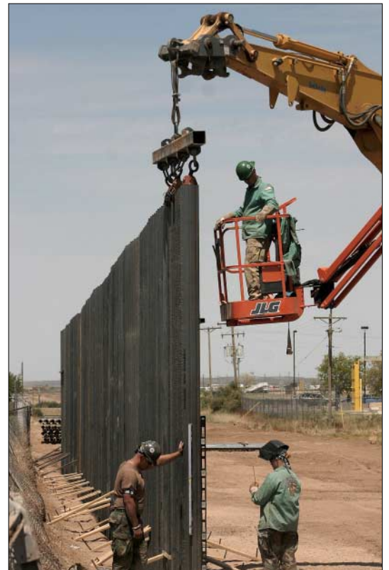
U.S. Army personnel install sections of the fence near Puerto Palomas, Mexico. U.S. officials expect to complete 670 miles of pedestrian and vehicle barriers by year's end.
